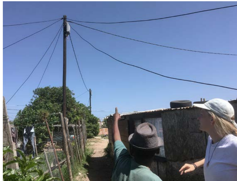
Khusta pointing out the electricity pole
